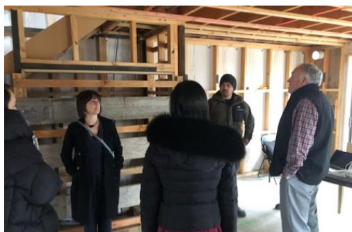
LEFT: Inspecting the inside of Pavitt St housing with members of St John of God Hauora Trust
